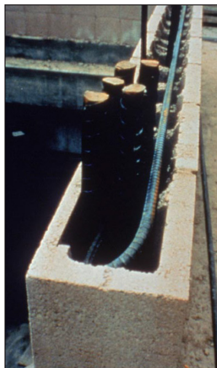
Figure 11 - Horizontal shear reinforcement is required to be anchored around vertical reinforcement with standard hooks for Special Reinforced Masonry Shear Walls (SRMSs). However, whether this is required on all horizontal bars in SMRSs is debatable. What is not debatable, is the congestion that can occur with significant vertical bars, lap splices, and horizontal bars with hooks in these potentially highly stressed locations.
