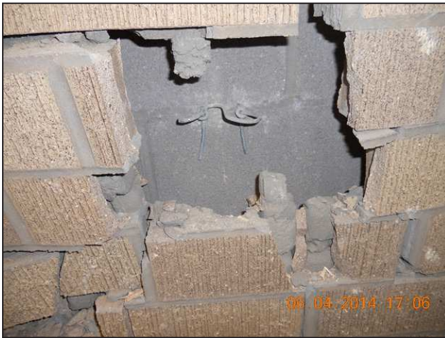
Figure 9 - Localized damage at the impact locations. Note the damage to the tie and veneer but no damage visible to the CMU face.
